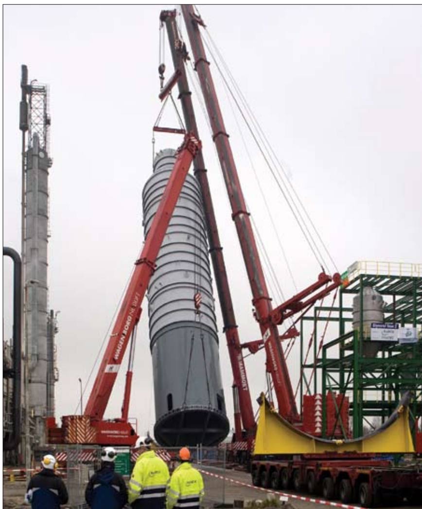
Placement of the purification column during the construction of a new biomethanol plant
